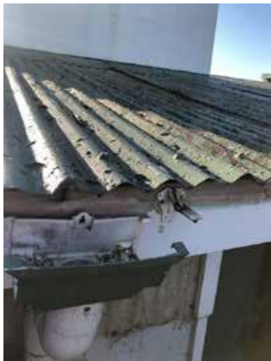
Roof and spouting requiring maintenance
