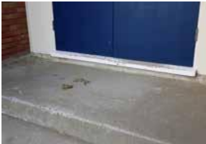
The door sill needs protection
