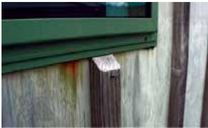
Plywood with no paint or stain protection
