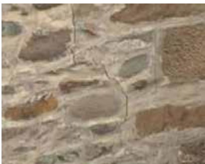
Cracking in stone wall
