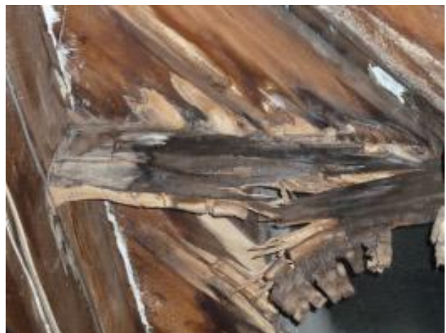
Damage from a large leak through the roof.
