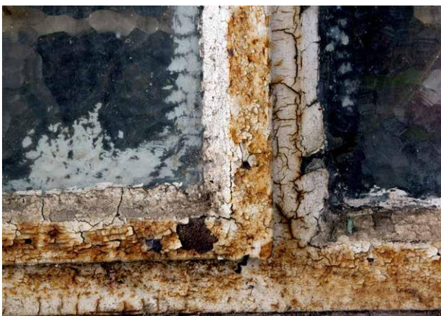
Severe corrosion on steel window frame
