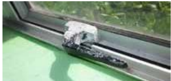
Surface deterioration on window hardware
