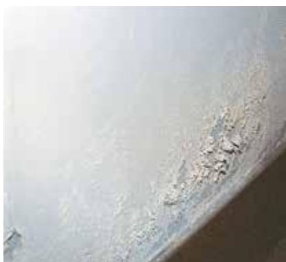
Signs of flaking and peeling paint indicating moisture in concrete wall
