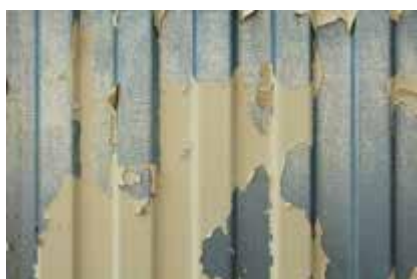
Paint peeling from metal cladding
