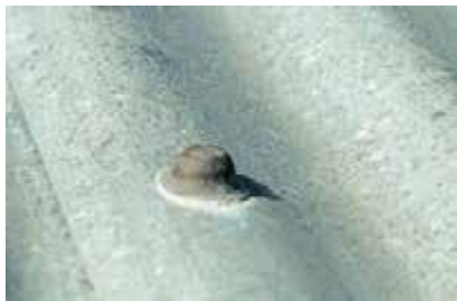
White rust around nail head
