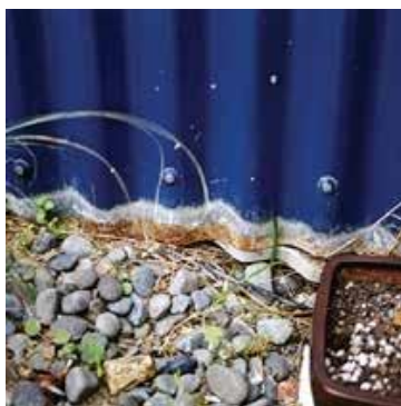
Corrosion to base of metal cladding that is too close to ground level
