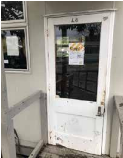
Broken handle to exterior door
