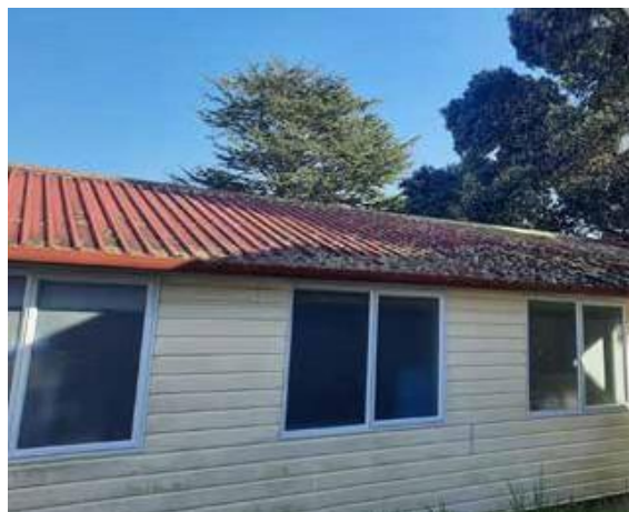
School building with lichen on the roof and mould on the wall cladding.
