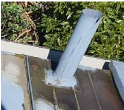
Corrosion of roof around penetration
