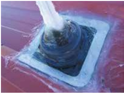
Roof penetration inadequately sealed
