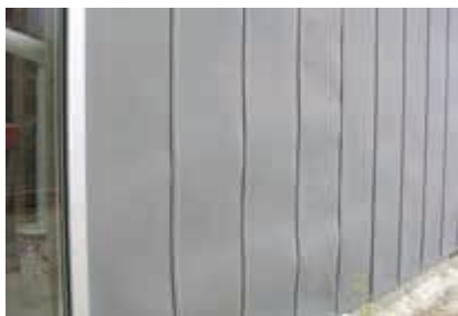
Metal cladding showing signs of buckling under thermal movement
