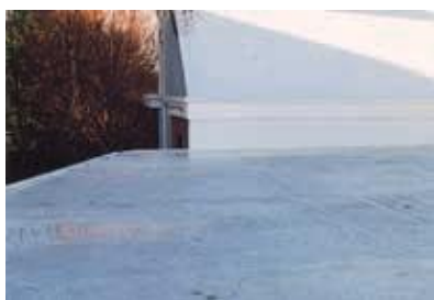
Insufficient fall to roof
