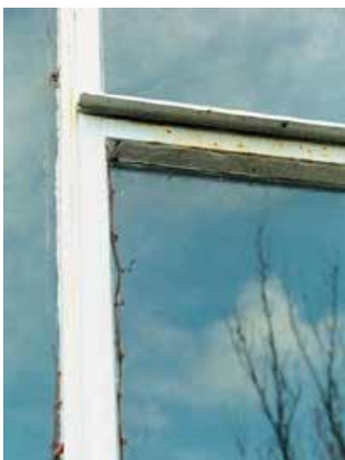
Signs of surface rust appearing on steel window frame
