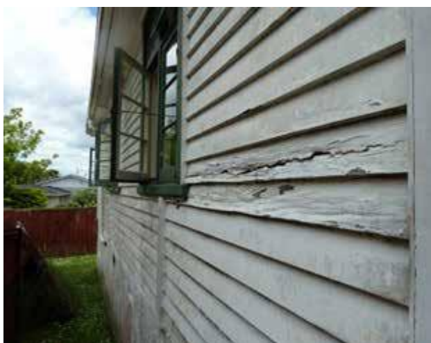
Severe rot in horizontal timber weatherboards
