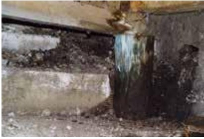
Piles showing signs of timber decay
