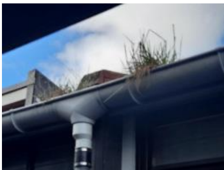
Vegetation blocking the spouting causes water to overflow and make the accessway below slippery
