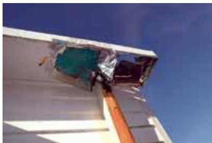
Joint failure in gutter
