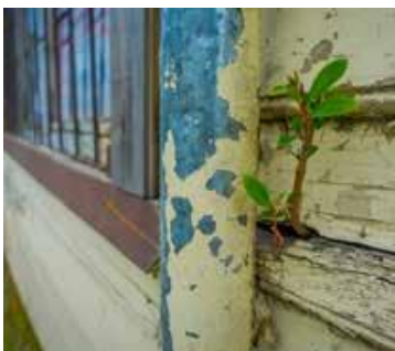
Plant growing in wall cladding
