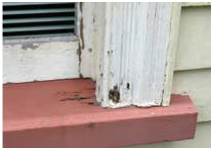
Timber window sill and facing cover board showing signs of rot
