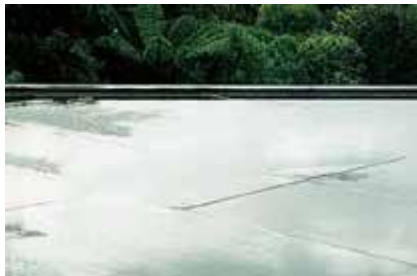
Water ponding on membrane roof
