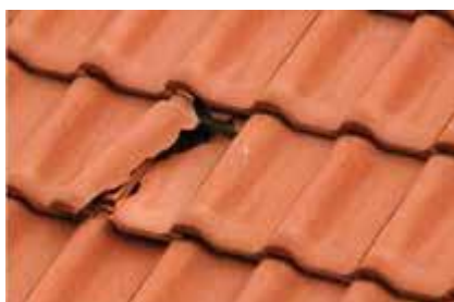
Cracked clay tile
