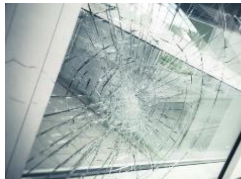
Impact damage to a glass panel
