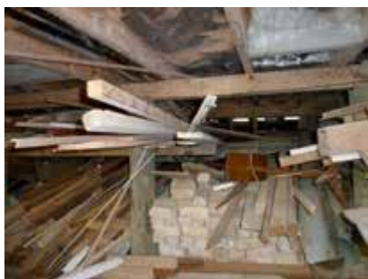
Items stored in the subfloor can restrict air movement
