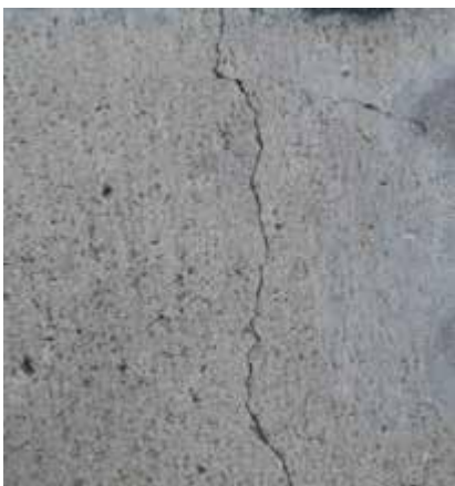
Hairline crack in concrete wall
