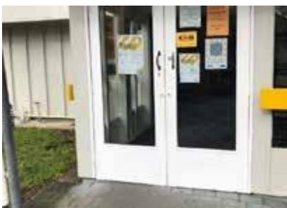
Timber door sill removed with paving built up to underside of door – potentially degrading bottom of door
