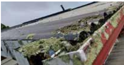
Lichen on gutter
