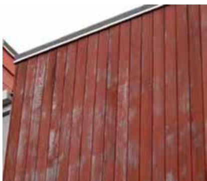
Plywood showing signs of needing to be painted
