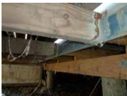
Rusting joist hangers
