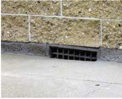
Subfloor ventilation is limited by concrete paving
