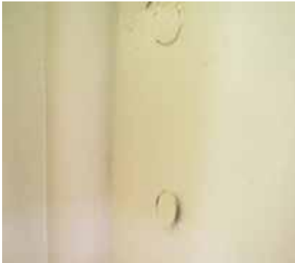
Nails popping through cladding
