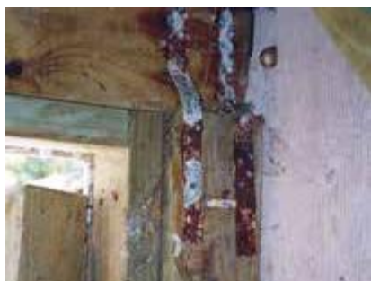
Rusted connections to jack stud framing.
