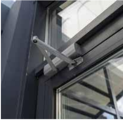
Self-closing door hardware to exterior door
