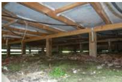
Lack of bracing to piles
