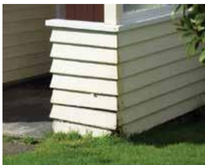
Cladding joint at mitre edge indicates failed junction
