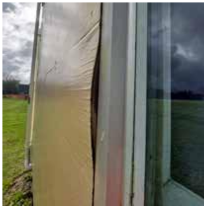
Cupping of plywood cladding
