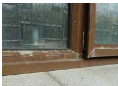
Coating failure on aluminium window
