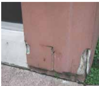
Cladding that is damaged and in contact with ground
