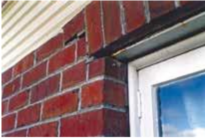
Header bricks detached from mortar indicating building movement or rusted steel lintel bar
