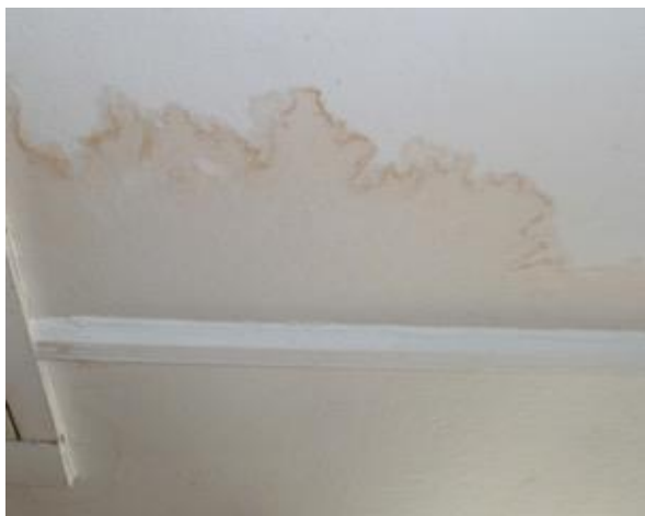
Evidence of a small leak in the ceiling or the start of a larger leak.
