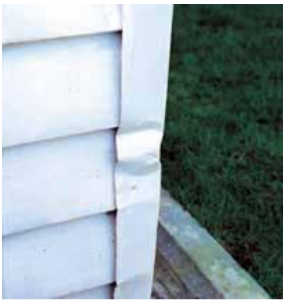
Impact damage to corner of metal cladding
