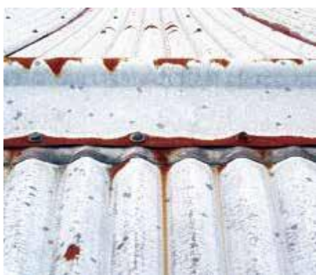
Red rust on galvanised roofing
