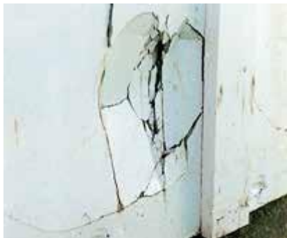
Impact damage to sheet – consider urgent repair
