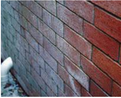
Efflorescence on brick veneer
