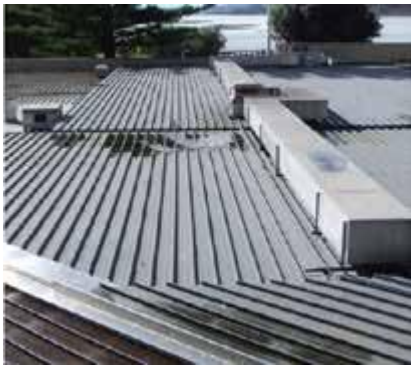
Insufficient fall causing ponding on roof
