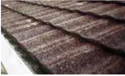
Loss of stone chip coating
