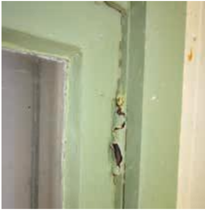
Corrosion of hardware can prevent windows from opening
