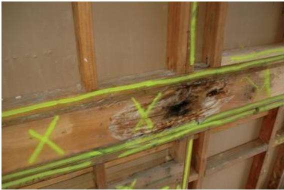
Evidence of a leak causing rot in timber framing
