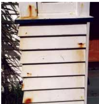
Rusty nail heads protruding through cladding
