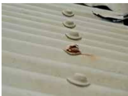
Corrosion of fixings
