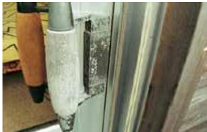
Surface deterioration on door hardware
