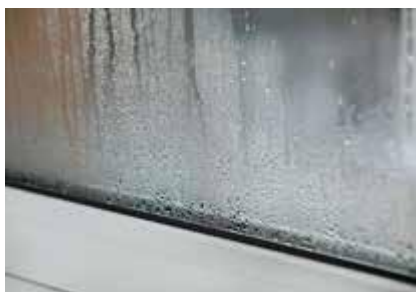
Moisture in double-glazed unit
