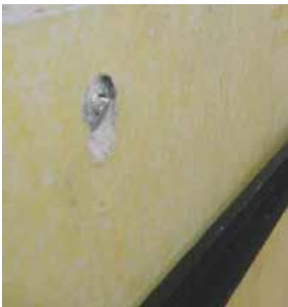
Signs of coating failure at panel fixing
