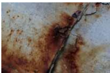
Severe rusting of metal surface
