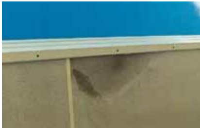
Soffit damage due to leaking gutter
