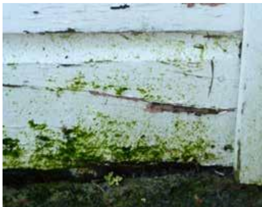
Degrading weatherboards at base of exterior wall
