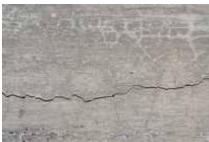
Cracked concrete wall in need of repair
