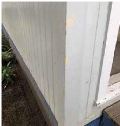
Dirt splashed up onto baseboards
