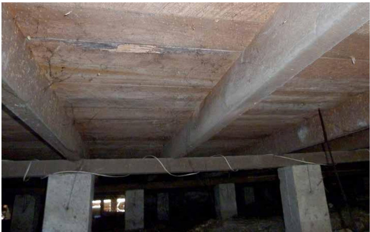
No subfloor insulation
