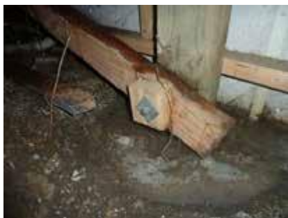
Subfloor brace too close to the ground and ponding water
