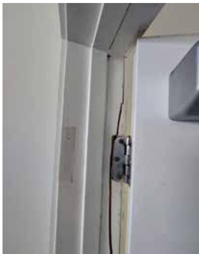
Damaged door jamb
