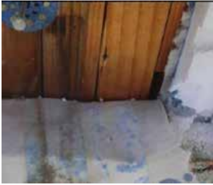
Impact damage causing failure of cladding system
