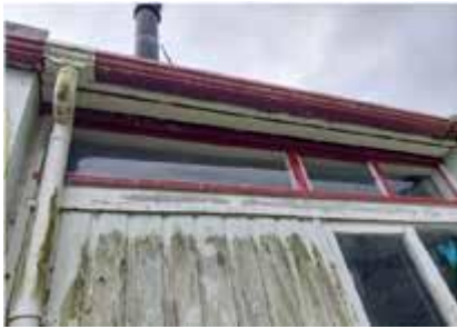
Spouting requiring urgent repair
