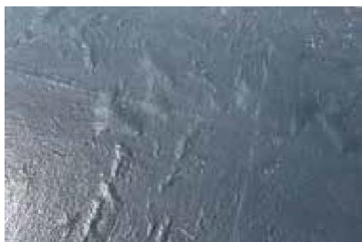
Bubbling under liquid-applied membrane
