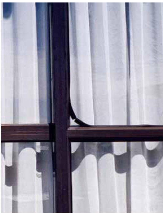
Failed rubber seals
