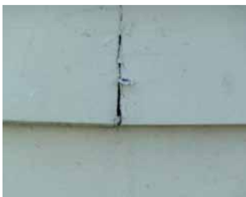
Crack appearing in weatherboard cladding
