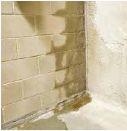
Basement wall showing signs of water penetration
