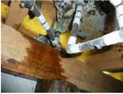
Leaking water pipe
